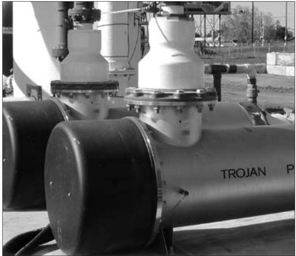
The Trojan UV-oxidation system at Stockton.
