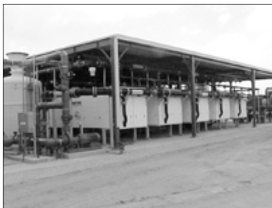
Microfiltration unit at the West Basin Municipal Water District.
