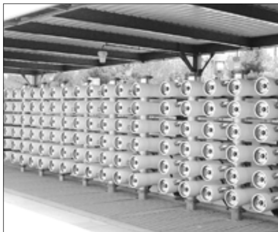
Reverse osmosis unit at the West Basin Municipal Water District.
