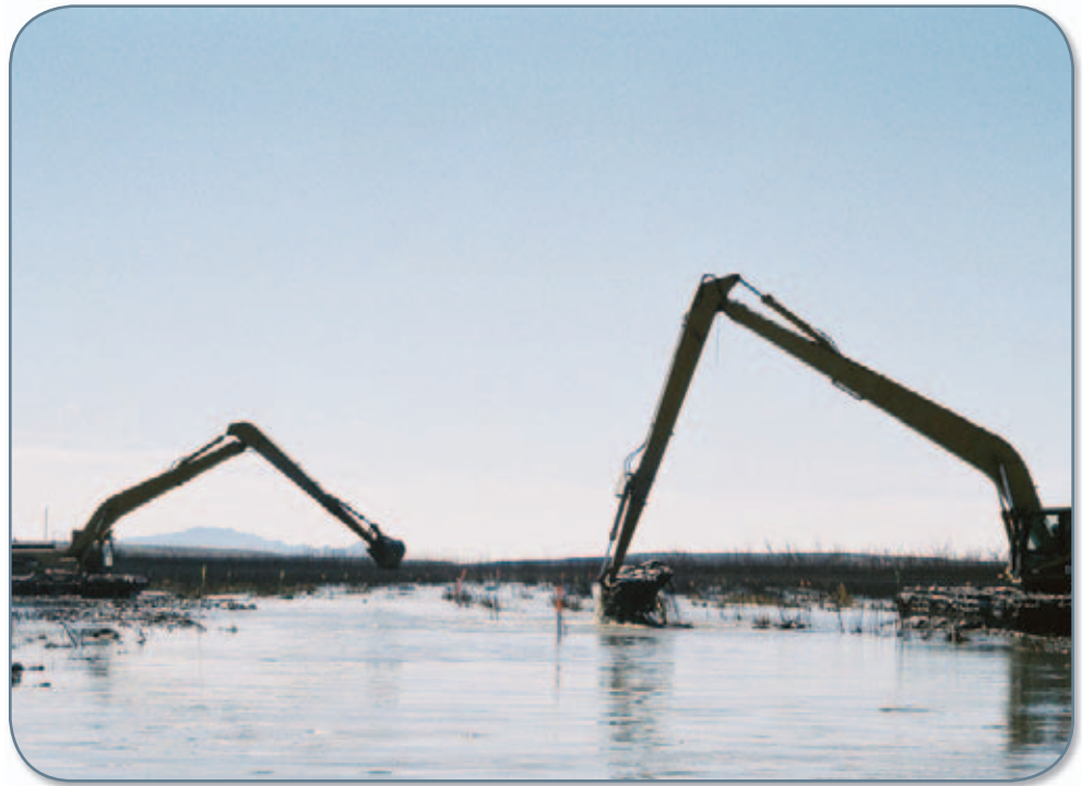
"Marsh buggies" or amphibious excavators, clear the channel through Elephant Butte Reservoir.
